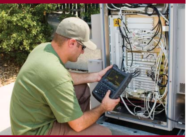
Figure 1b. FieldFox directly connected to a feeder line on a wireless communication system
